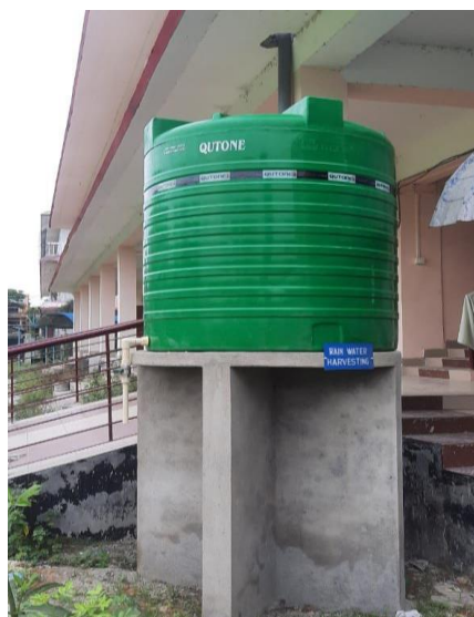
Photo 3: Rain Water Harvesting Unit
